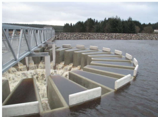
Back Esk Reservoir spillway – PKW made of prefabricated concrete elements (Courtesy of Black and Veatch Ltd)
